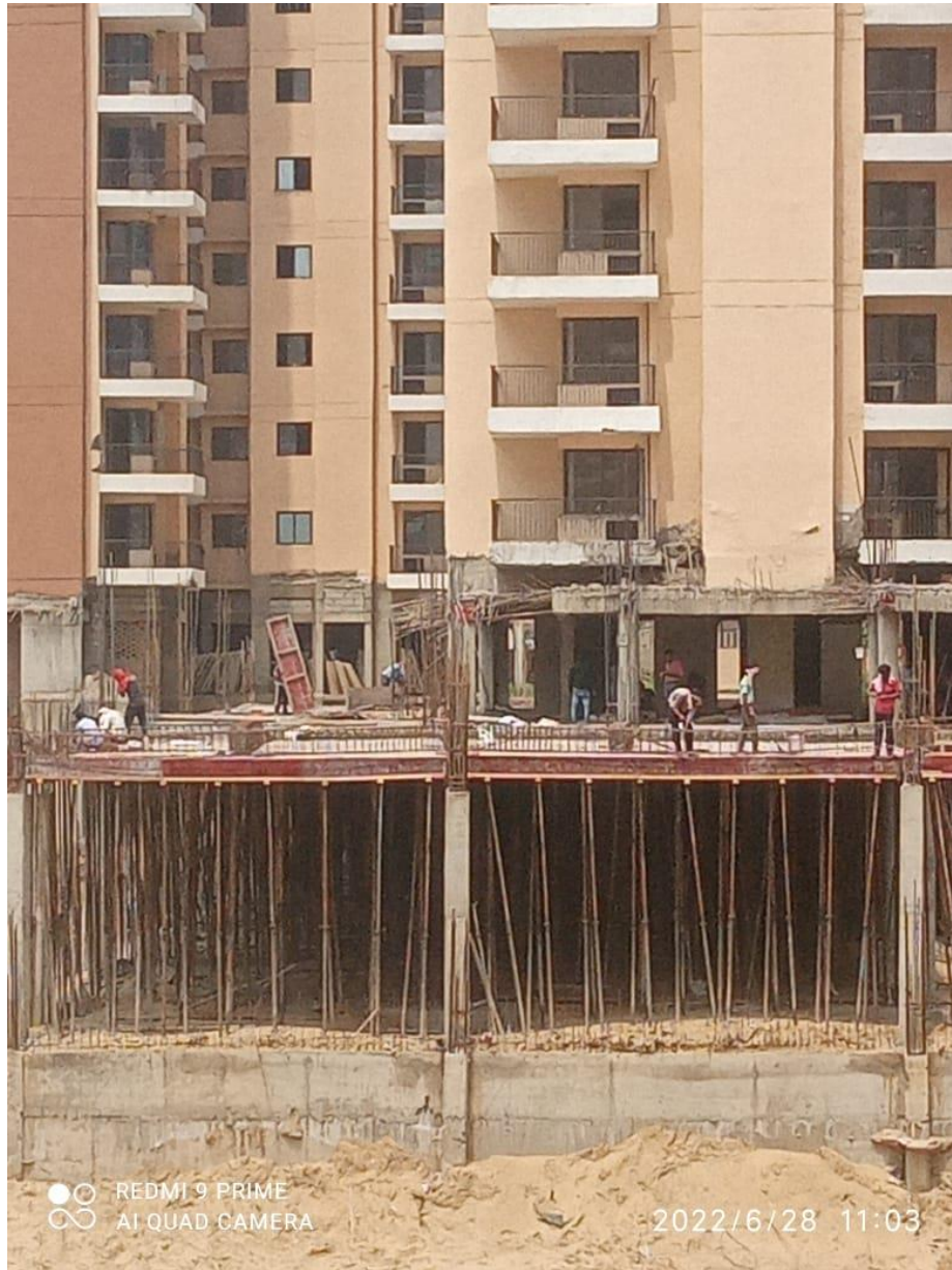
Non Tower Area near Tower C, Slab shuttering work is in progress
