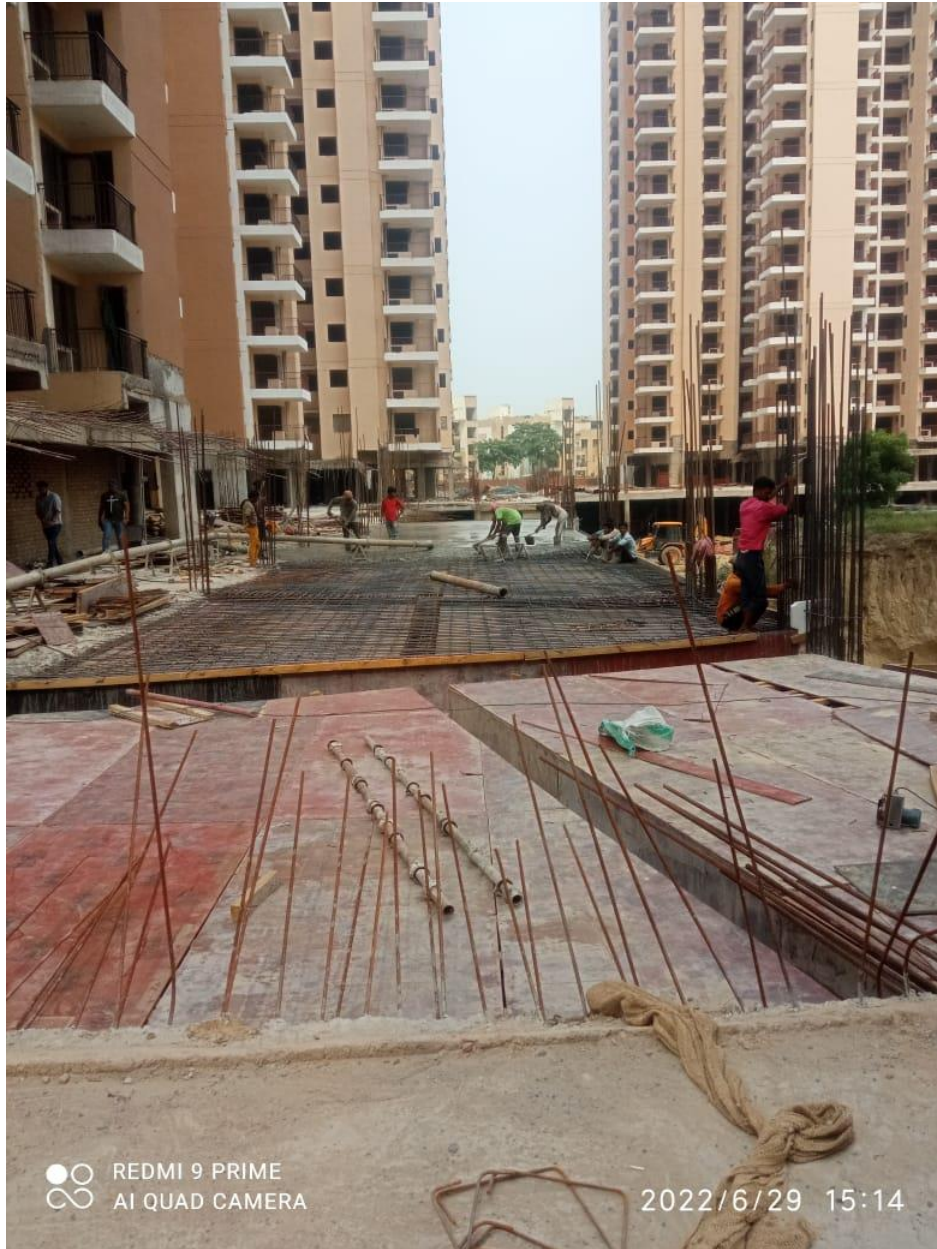
Non Tower near Tower B and C : Slab concreting work is in progress
